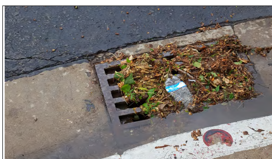
Storm water drain overwhelmed by debris. Causes street flooding.
