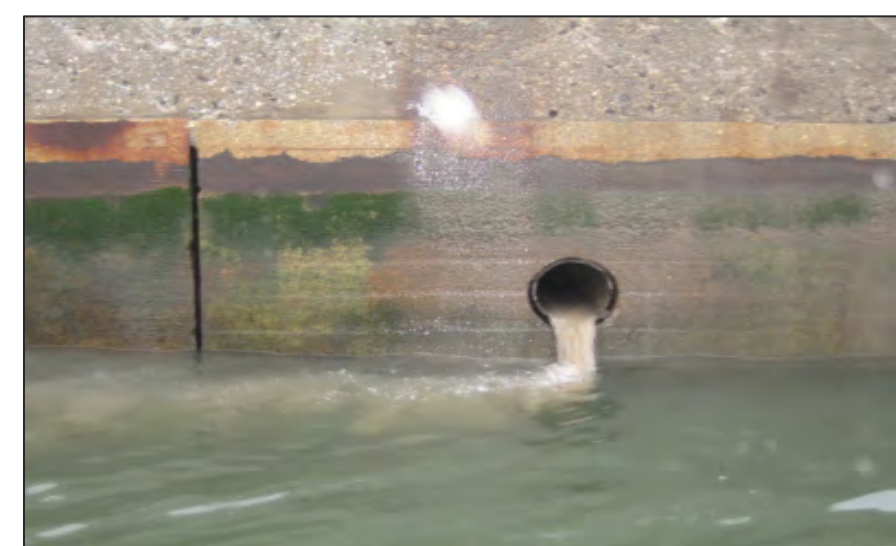
Combined Sewage Overflow (CSO) into receiving water body.
